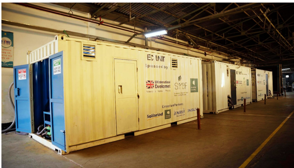
Figure 2. The SMEP pilot containers deployed on site in Bangladesh - funded by SMEP
