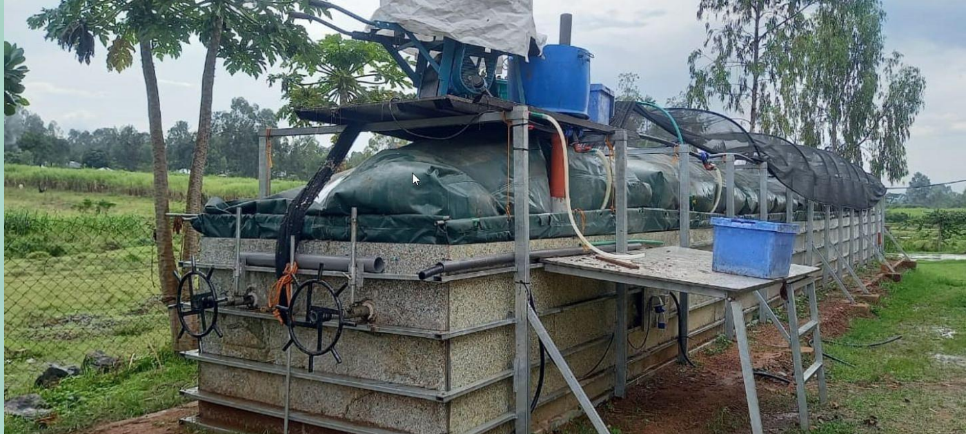
Photo 12: T-Rex 100 M3 biodigester installed at Rio Fish
